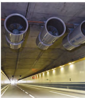
Smoke extractor in a tunnel
